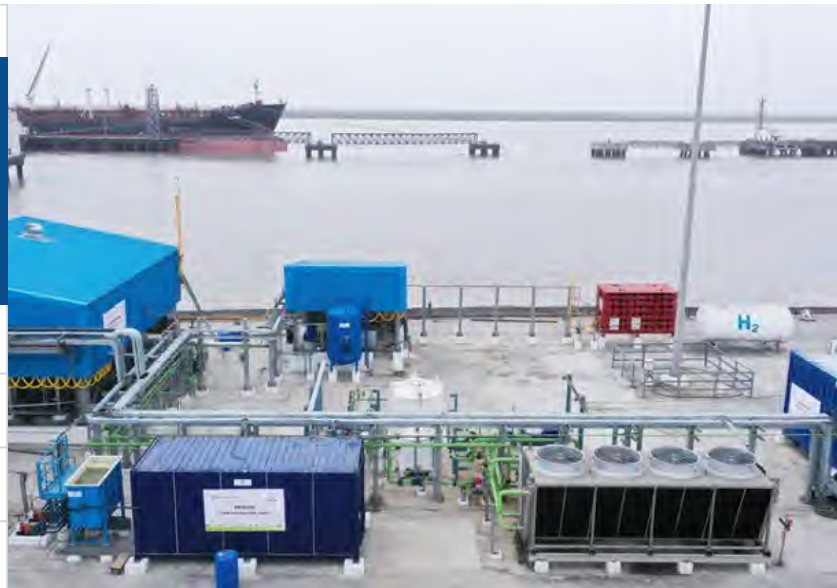
1 MW Green Hydrogen Plant for Deen Dayal Port Authority at Kandla, Gujarat commissioned by LTEGL
